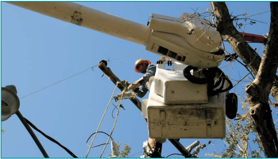
A lineman from Indianapolis Power & Light installs a new insulator in Lake Charles, Louisiana, on October 5, 2005. Downed utility lines had to be replaced before residents could move back in. Photograph by Marvin Nauman/FEMA
